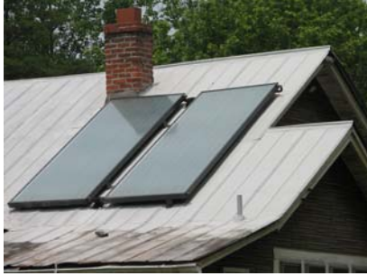
High Tech Panels on a Low Tech Farmhouse: An FLS Energy solar installation at Thatchmore Farms.
